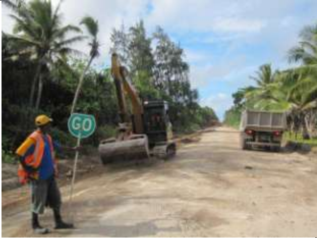
Undercut and side drains being excavated near Eton Bridge just North of Eton Village
