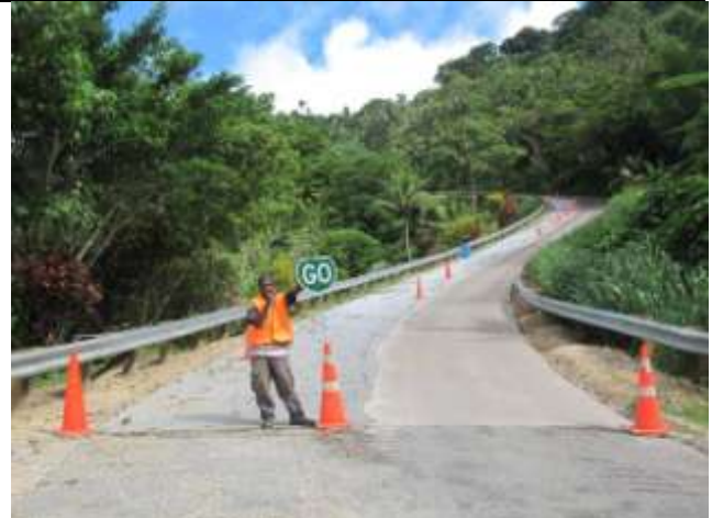
Klehm's Hill, with the concrete roadway complete. Drainage, guardrail and finishing off work is now underway.
