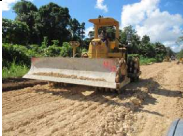
Santo: Compacting and shaping pavement near the 39 km mark, South of Hog Harbour.
