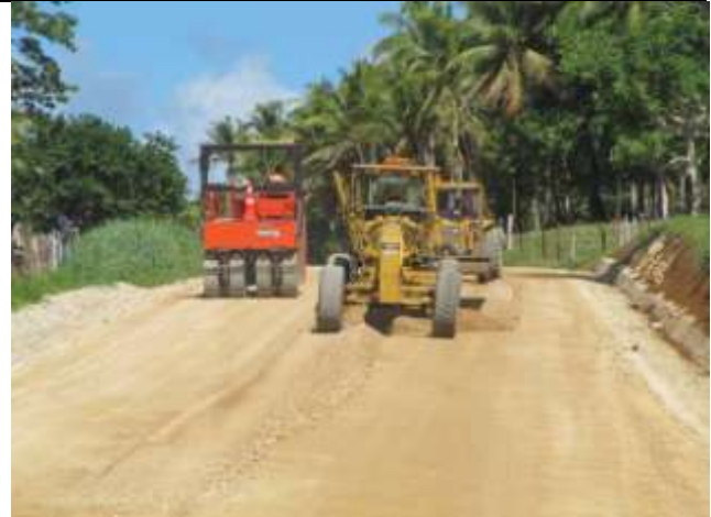
Efate – final trimming and shaping of the pavement in preparation for sealing at the 50 km mark near Ekiye Village.
