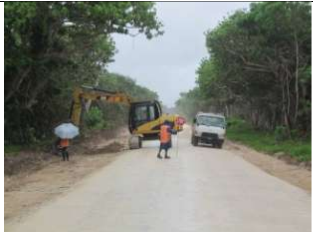
Digging drains on a wet day. Downer EDI Works Vanuatu staff work through a rain shower near Dry Creek.
