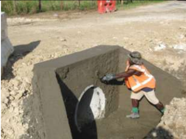
Finishing touches to the final 750 mm diameter culvert on Efate. Fred Kai plasters a headwall
