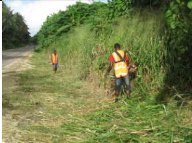
Efate: Clearing vegetation re-growth from the table drains near Safaki. This work is being done by Downer workers, the next clearing work will be done using community contracts with the villages along the road.
