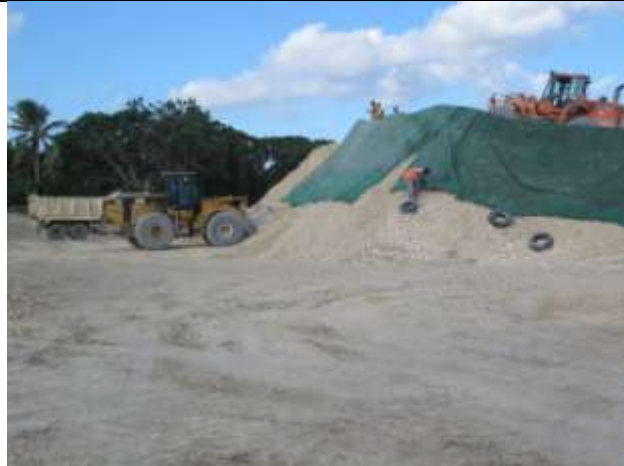
Efate: Last load for the day. The Cat 966 loader operated by Joel Kalsal loads the last truck for the day as other quarry workers place the covers to keep the stockpile dry overnight.
