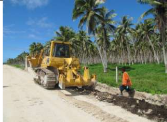
Efate: A bulldozer ripping the ground to break up large rocks so that the table drains can be excavated near the 85 km mark. The D 155 A machine is operated by Jacky Kaltapiri while Alex Muramur provides guidance.
