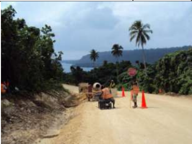
Santo: Rock lined drain under construction on the Champagne Beach Hill. This work is now nearly complete.
