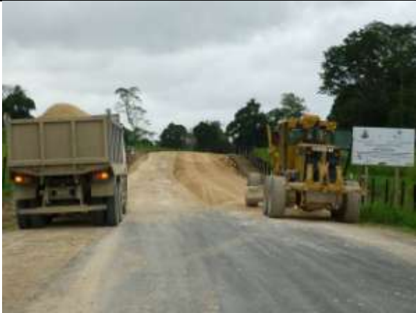
Efate: Starting at the End: Downer plant at the end of the Japanese Road working back towards Erueti to utilise drier pavement material. Only 5 km of old road remain to be overlaid.
