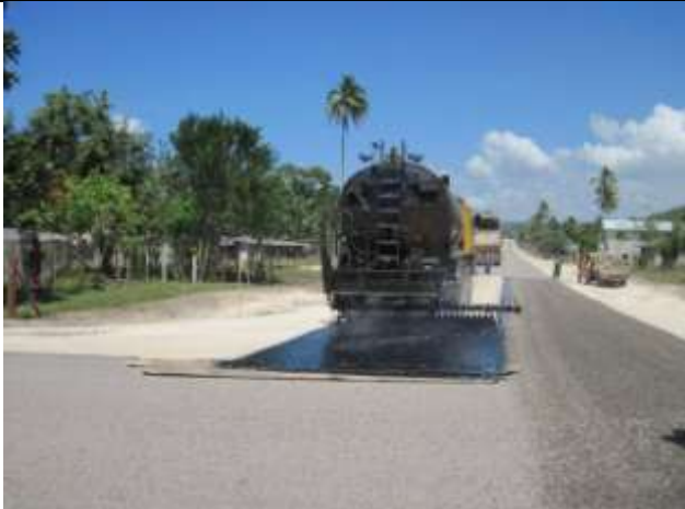
Spraying the final section of first coat seal on the Santo East Coast Road in Port Olry.
