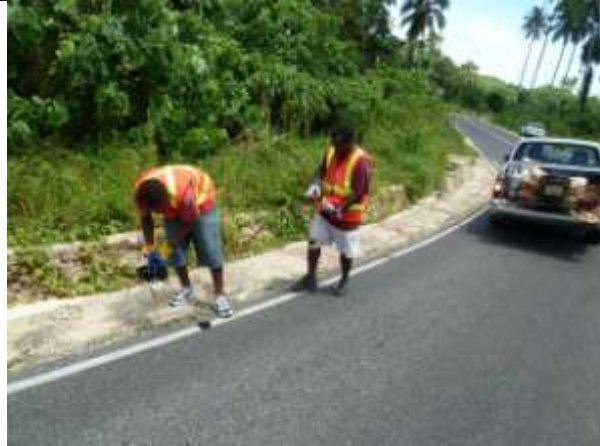
Trevor Lenga and Sity Jack laying red pavement markers on a corner near Champagne Beach.
