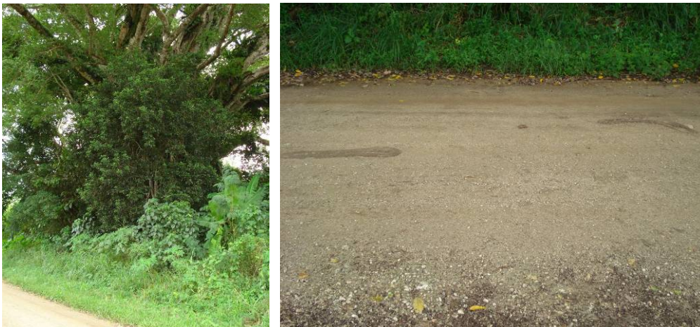
Figure 3: Nabanga Tree at 74 showing visible roots in road carriageway
