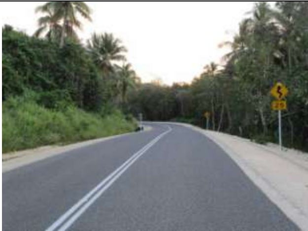
Getting ready for the Hand-back Ceremony. A completed section of road on Efate with safety signs in place and line marking completed.
