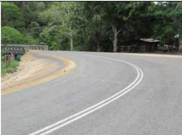
The new seal reaches the Epule Bailey Bridge – 47 km from the start of the Project on Efate
