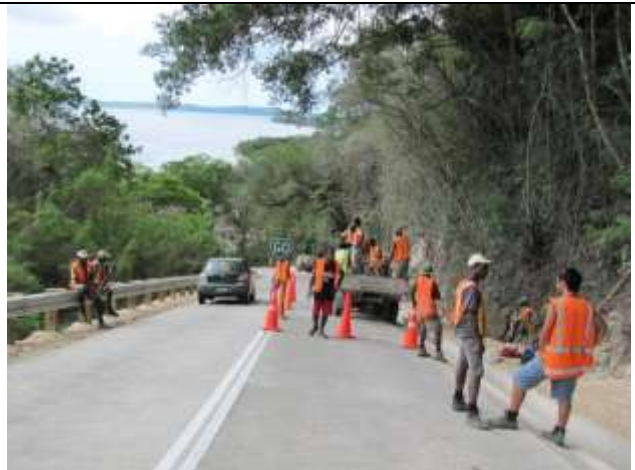
Final tidy up on the Lelepa Hill concrete pavement site. Downer Cadet Matthew Smith (right) discusses work with subcontractor M A Builder's representative
