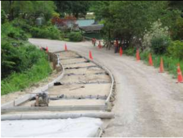
The first strip of concrete pavement reaches the bottom of Klehm’s Hill. Traffic is now using the concrete pavement near the top of the hill. Overall this work is nearly half finished.
