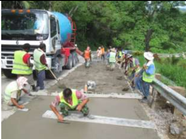
Klehm's Hill – the end in sight, an agitator truck discharging as the work crew compact and finish the concrete near the base of the hill. The major concrete work is expected to be finished this weekend. There will then be a 7 day period for the concrete to gain strength before traffic is restored to two lane flow.
