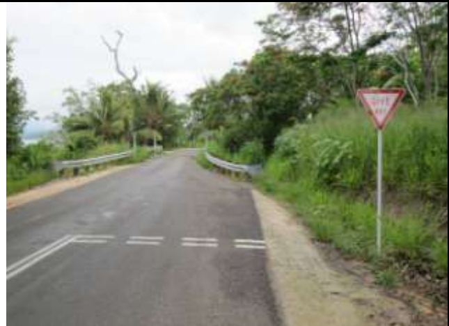
Give Way sign and road marking advising which traffic should give way and where they should wait until the road is clear where it is only one lane wide. If a vehicle has moved beyond the road markings and a second vehicle approaches from the other direction then the second vehicle should give way.
