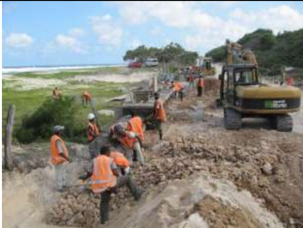
Downer EDI Works staff constructing a gabion basket wall on the downstream side of the new triple barrel culvert at Dry Creek (just South of Eton).
