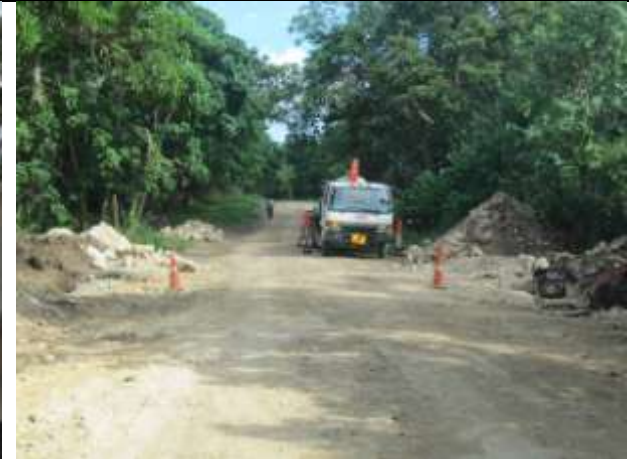
Santo: Installing a culvert just North of Hog Harbour on the road to Port Olry.
