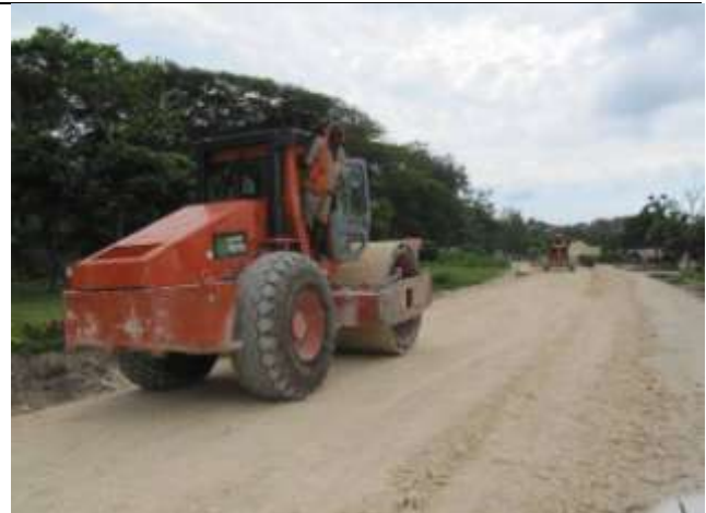
Efate: Downer roller operator Edward Tasaruru compacting the pavement on the outskirts of Eton village.
