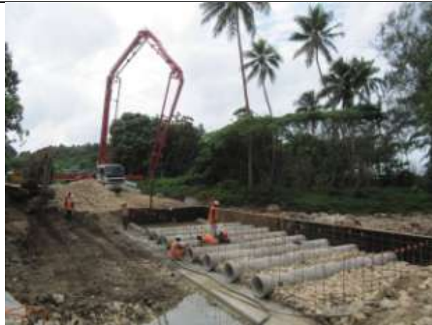
Efate: New pipes laid for the Neslep Crossing at Elownea Bay, with the concrete pump set up in the background ready to start work.
