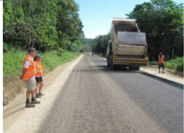
Downer New Zealand General Manager, Commercial Operations Jeff Oldman and Engineering Cadet Amanda Taylor observe sealing underway near Ekipe.
