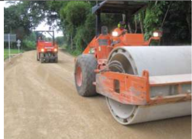
Final preparation for sealing in Epau village. These rollers are operated by Malcom Arthur (left rear) and Joseph Noveil (right front).
