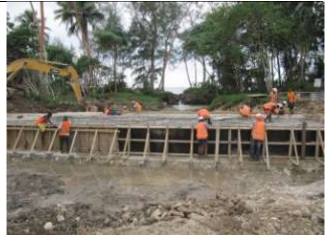
The Neslep Crossing at Elownea Bay, with the work crew placing formwork and reinforcing steel ready for a concrete pour.
