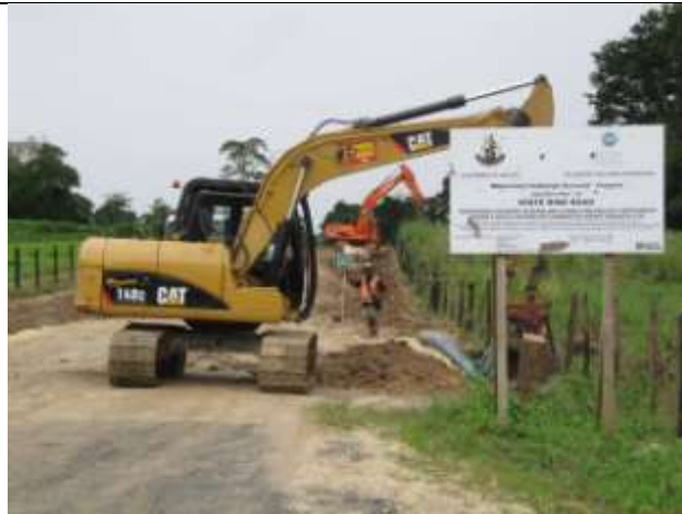
The last clearing and widening. Downer excavators connecting the last section of new drain into the existing drains at the end of the Japanese Road.
