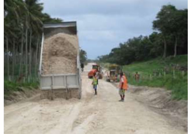
Efate: Spreading coral aggregate and checking pavement levels near the 85.8 km mark. David Jackson controls operations.
