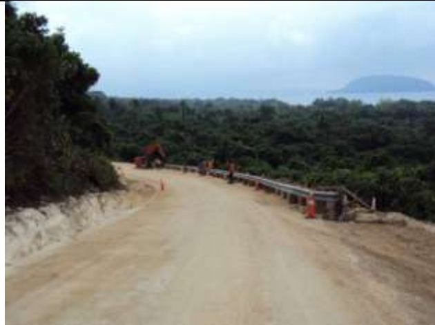
Santo: Road widened and guardrail under construction on the hill above the Champagne Beach turnout.
