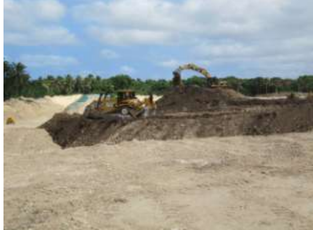
Efate: Progressive rehabilitation at Nangas Quarry. As coral is removed the excavation is being backfilled with stockpiled topsoil.
