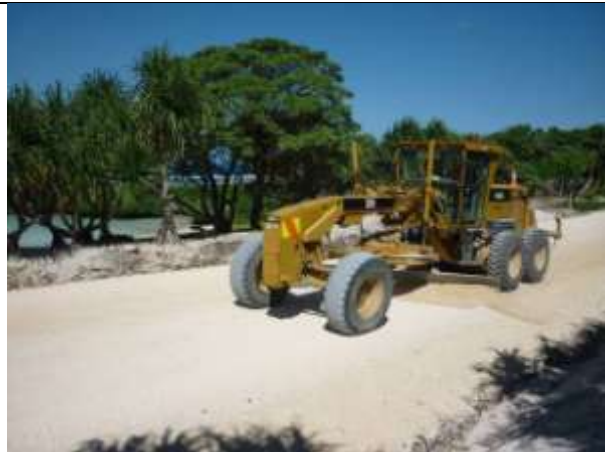
Preparing the pavement surface for sealing. A Downer EDI Works Vanuatu grader trims the road near Pesal's Beach.
