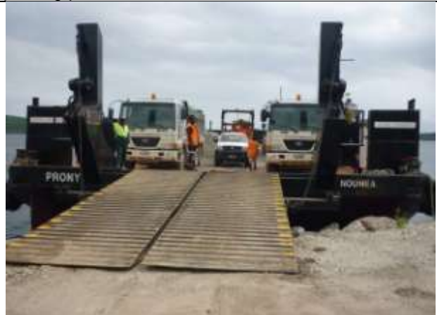
A loaded barge about to leave for Santo carrying additional equipment so that preparations to seal the remaining length of road can commence.
