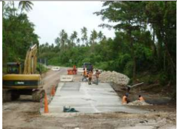
The Lakensua Floodway after the concrete was poured. The workers in the right foreground are placing protective reno mattress baskets
