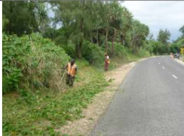
Downer EDI Works crew carrying out planned routine maintenance work in one of the sections Taken-Over by The Employer – in this case trimming vegetation near Onesua.
