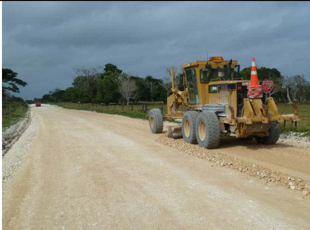
Final trim of the pavement near the 87 km mark at Erueiti to get it ready for sealing.
