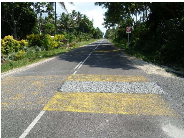
Speed calming trial at Paonangisu. A one metre wide band of very large size sealing chip in the centre of the yellow patch is intended to make a rumble sound as vehicles travel over it.
