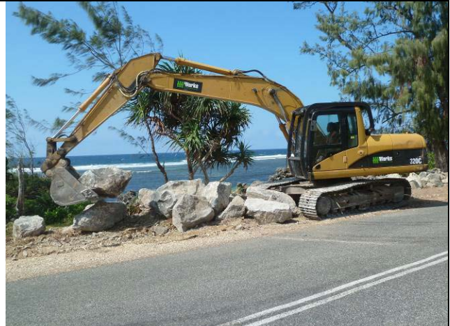
A Downer excavator operated by Kevin Ruben gently places basalt rip rap to improve the coastal erosion protection at Onesua.
