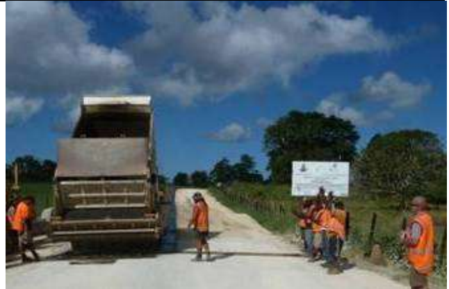
Cheers and applause as the truck placing the black stones reaches the Japanese Road. Sealing subcontractor Seaview Holding's General Manager "Nono" Cassart on left of truck and Downer Surfacing Supervisor Clinton Thombs on the right monitor the application of the black stones.
