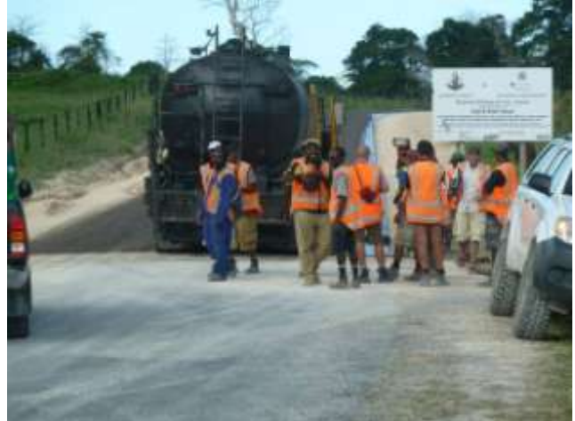
Downer workers gather as the last of the first coat seal bitumen is sprayed.
