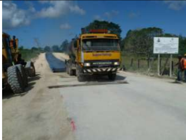
The new seal meets the old at the end of the Japanese Road. The first coat sealing crew reach the end of the Project length at the 92.6 km mark near Rentabao.
