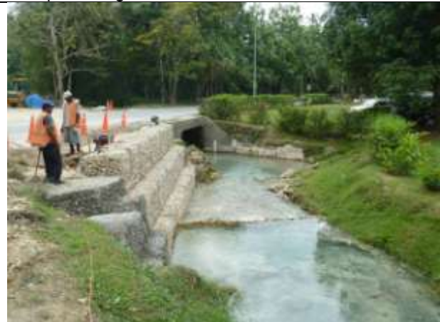
The nearly completed gabion basket protection to the road adjacent to the Mele Cascades.
