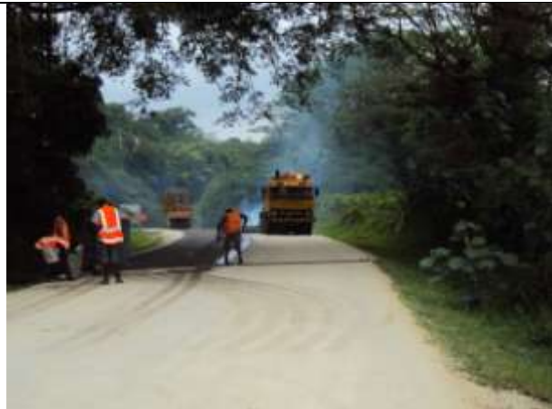
Sealing team near the crest of the Manioc Hill on the Santo East Road.
