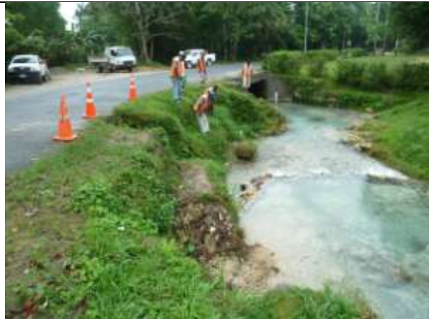
A Downer crew inspecting the gabion basket site at Mele Cascades prior to starting work.
