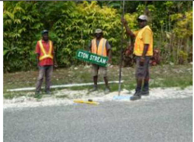
Jeffrey, James and Manau from subcontractor MA Builders installing signs in the Eton area.
