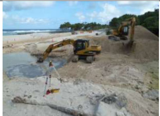
Downer hydraulic excavators dig the hole for the new box culvert at Dry Creek.
