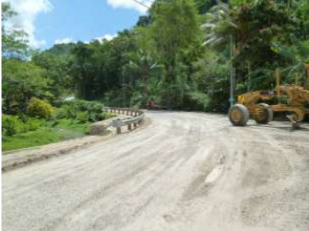
Starting work on the short section of pavement at the base of Klehm's Hill.
