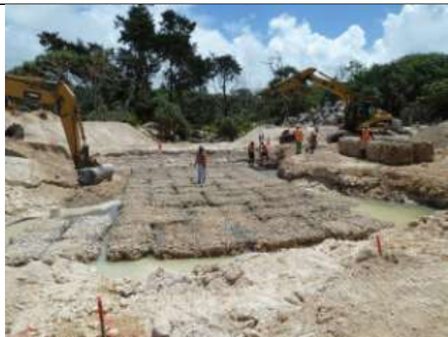
Constructing the gabion basket foundation raft for the Dry Creek box culvert.
