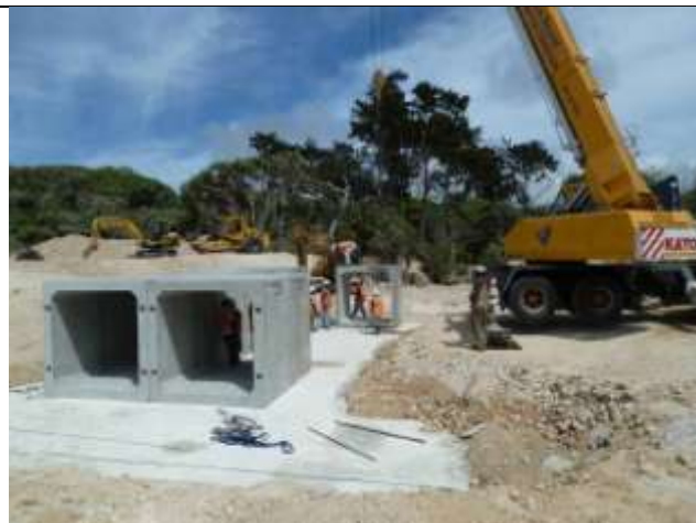
The crane from Pierre Brunet Enterprise Generale lifts the concrete box culvert units into place at Dry Creek.
