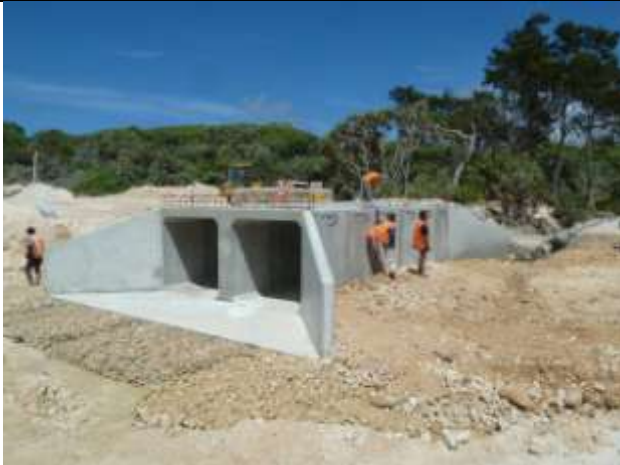
The Dry Creek Box Culvert immediately after the formwork for the concrete wingwalls was removed.
