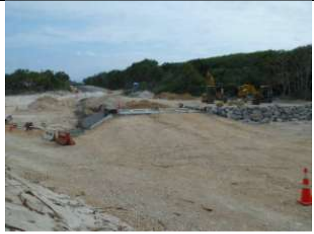
The site after most of the backfill has been placed around the new structure with the road embankment almost up to the top of the concrete units..
