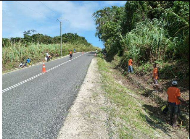
Efate Ring Road: Mangaliliu villagers carrying out work for one of the PWD organised Community Maintenance Contracts.
