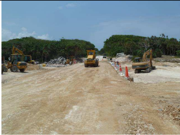
Efate Ring Road: Constructing the pavement over the new box culvert at Dry Creek.
